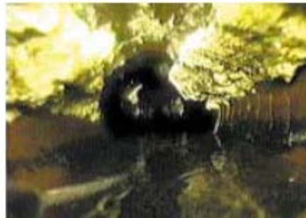
Figure 8: Grease Buildup Inside Sewer Pipes
